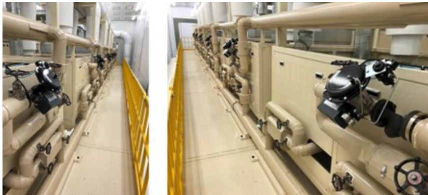
Photo of sliding gate valve in customer installation
